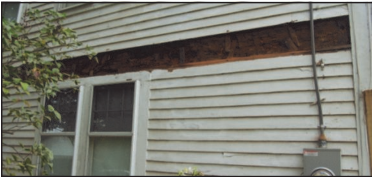
Repair work necessitated uncovering the south end girt - a large hand hewn beam from the original 1714 construction.
