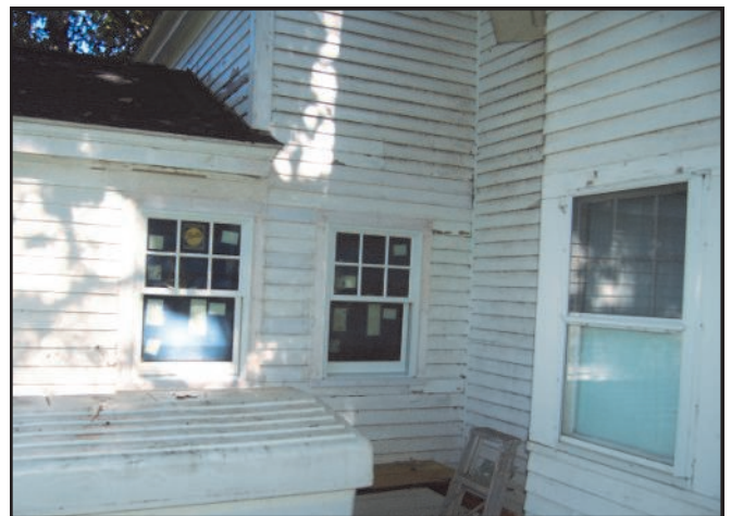
New kitchen windows have similar design and trim to original window (right).
